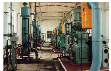
LW-20/25-X oil free piston air compressor unit (glass factory)
