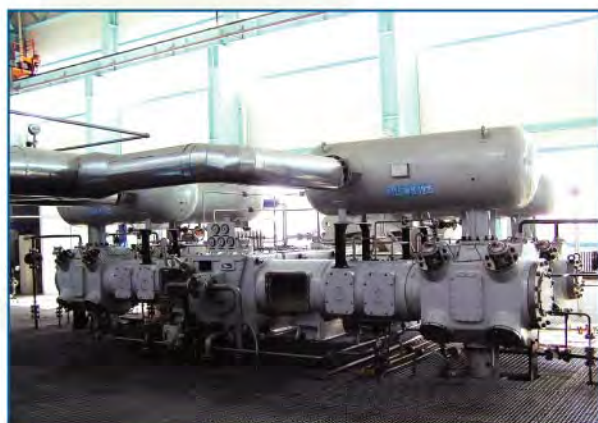
4M25 hydrogen compressor
