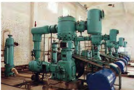
LW-22/7-X oil free piston air compressor unit (cement factory)
