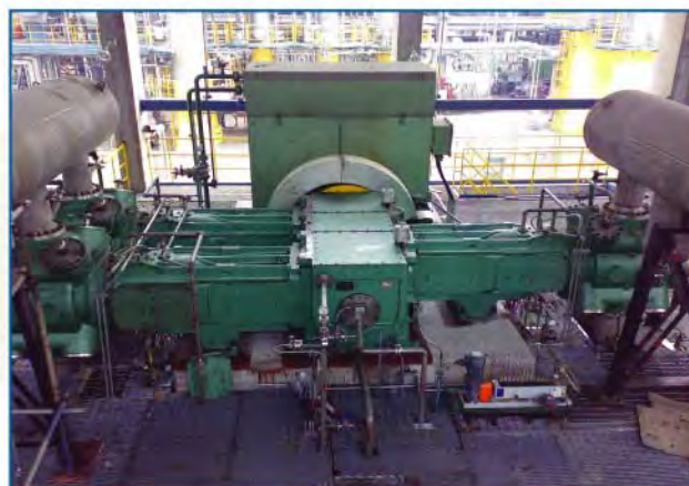
KR60-3 compressor installation
