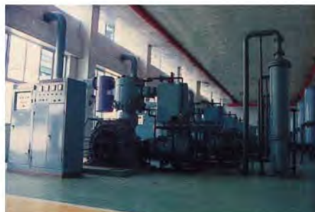
LW-40/10-X oil free piston air compressor unit (electronic factory)
