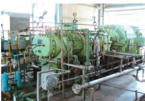
Screw cracked gas compressor
